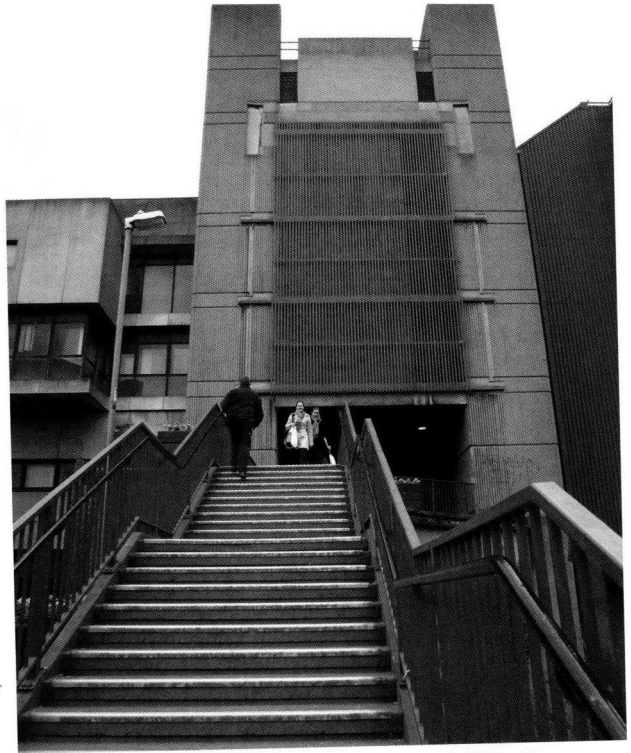
Fig. 13 Scar of planned connection to unbuilt section, photographed in 2013. Photograph by Peter Larkham
